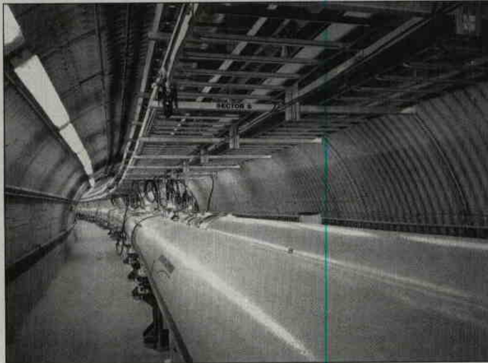
RHIC magnets, a view inside the RHIC ring tunnel. Photos courtesy of Brookhaven National Laboratory.
