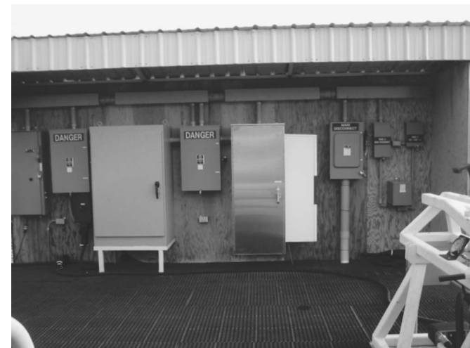
Fig. 3. Electrical supply for the motor testing
