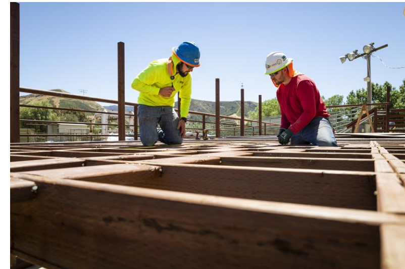
Students Tim Smith and Ryan Fiorio work together to complete decking layout.
