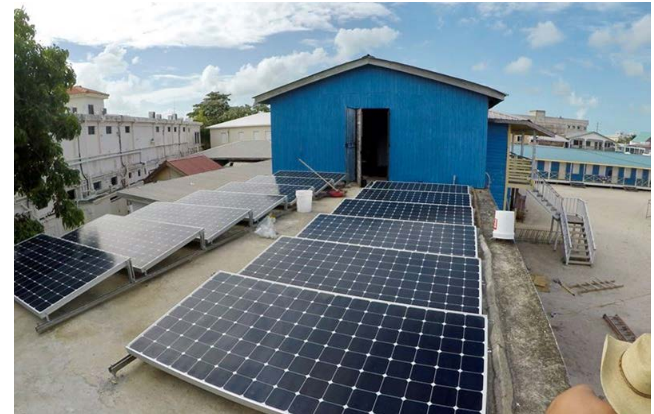
Figure 4: Completed PV layout
