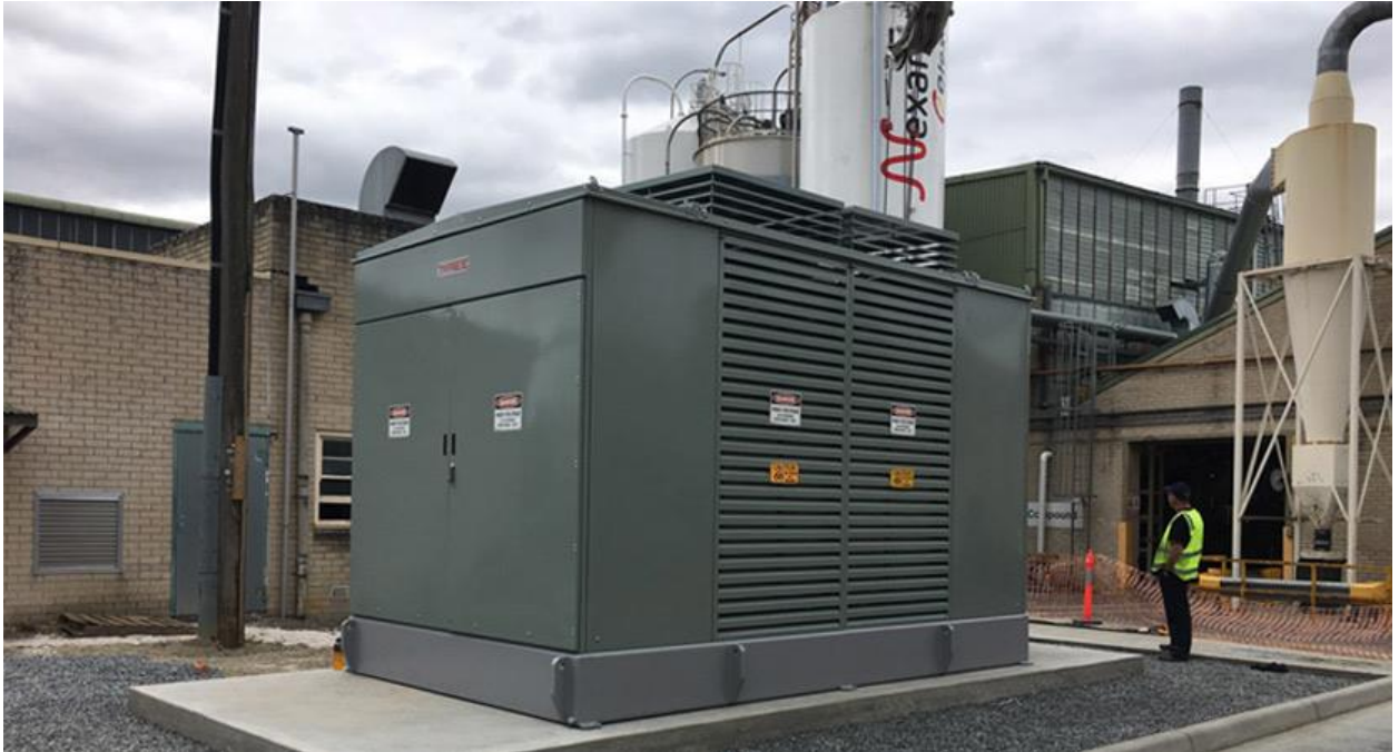
Figure 2.4.2: REFCL Isolation Bank Used in Australia [18]
