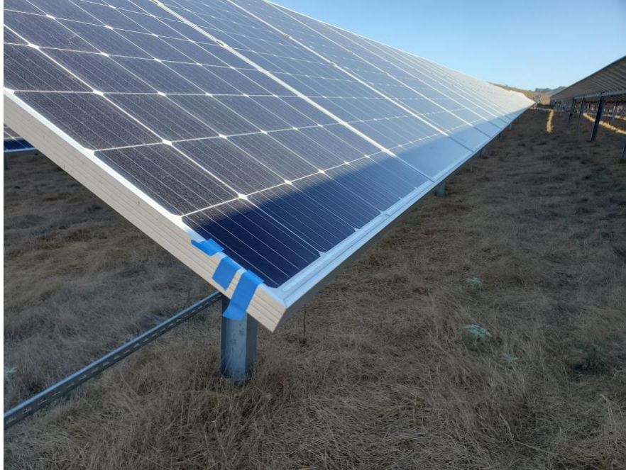
Figure 4.2 Actual shading seen at the Gold Tree Solar Farm. The shade shape is a triangle extending across the row. As time passes, this triangle grows in area.
