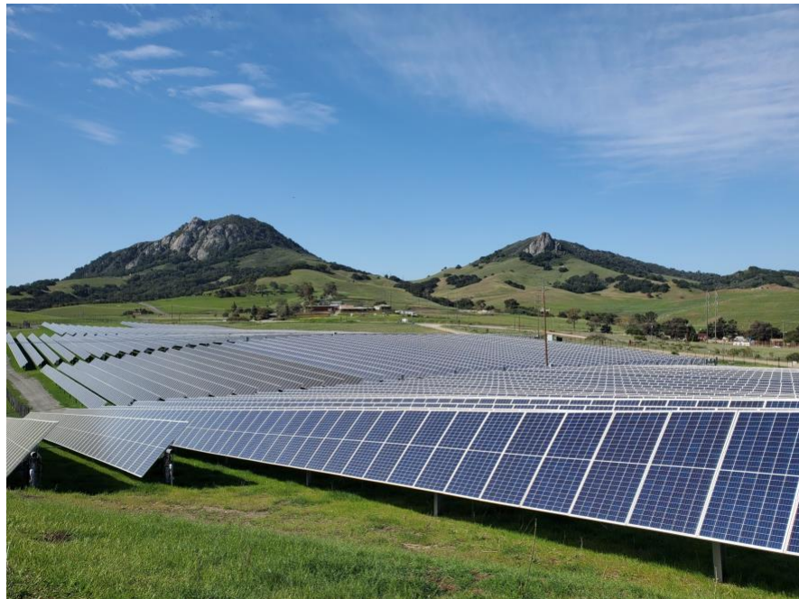
Figure 2.1 The Gold Tree Solar Farm
