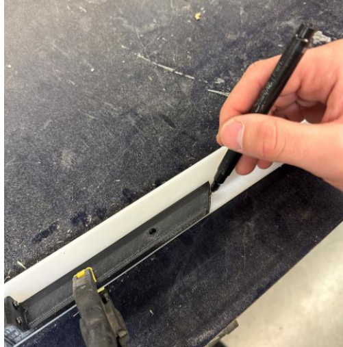
Figure 26 – Using a marking jig to mark the length and angle of one end of the plastic angle siding.
