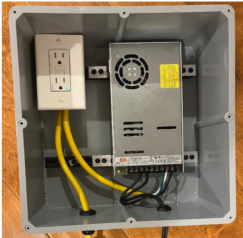
Figure 11 – GFCI and LRS-600-36 in waterproof box (lid off).
