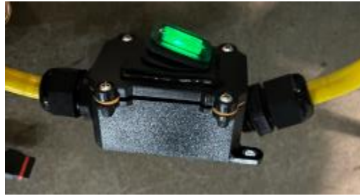
Figure 138 – Power supply’s green switch flipped to the on position.
