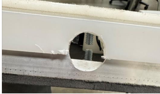
Figure 42 - Shows both the oversized bolts and the hole in the side supports for the wires to pass through.
