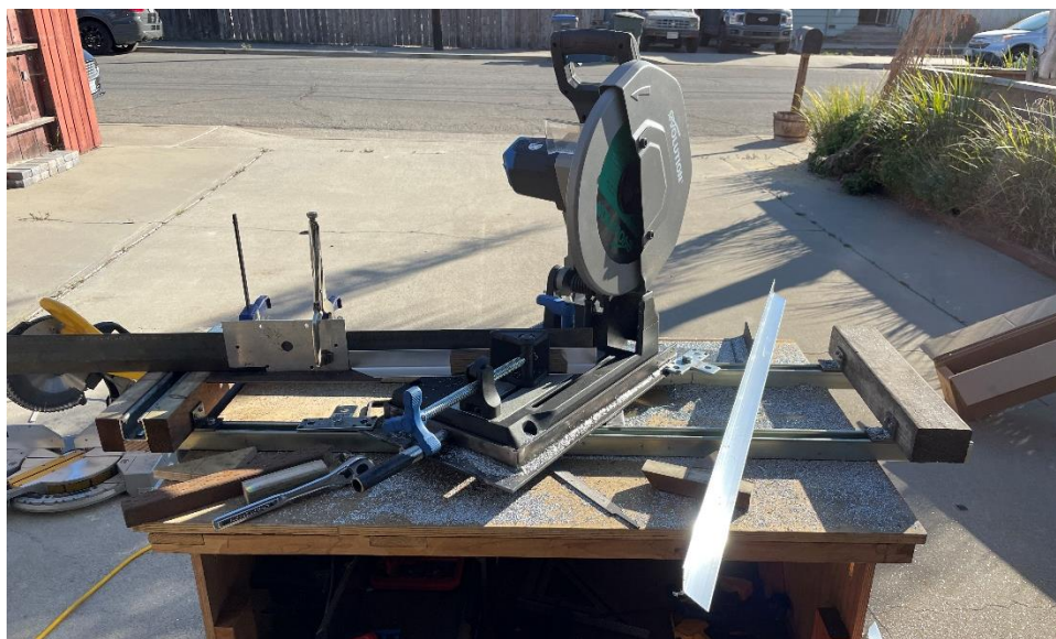
Figure 50 – Saw was repositioned to a 52.5 degree angle to complete parts 122C and 122B.
