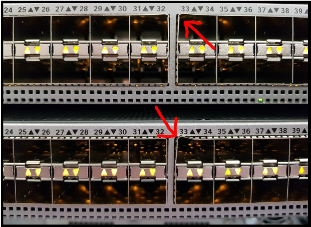
Figure 9: Nexus 9200 Chassis with Damaged Front Ports
