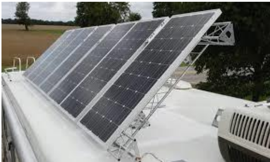
Figure 2: Solar panels atop jobsite trailer.
