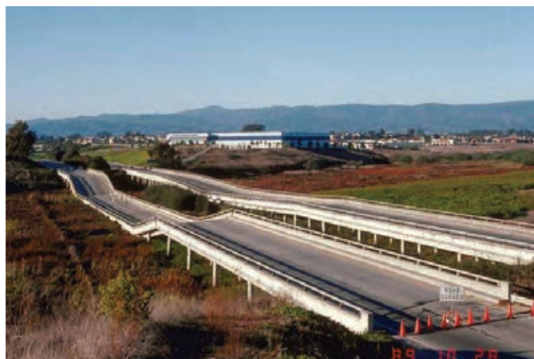
Figure 2: Damage to Highway 1 near Watsonville after the Loma Prieta Earthquake. Extensive damage to this critical roadway severely impacted earthquake recovery. (J.C. Tinsley, United States Geological Survey)
