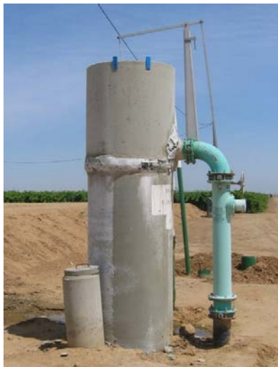
Figure 4. Assembled float mechanism on a turnout at Delano-Earlimart Irrigation District – without the recommended manual pressure reducing valve, or pressure relief and vacuum relief valves.
