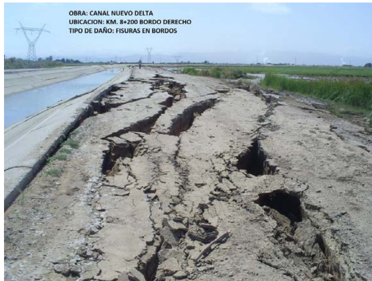
Figure 9. Fissures in the embankment road. Photo courtesy of CONAGUA.
