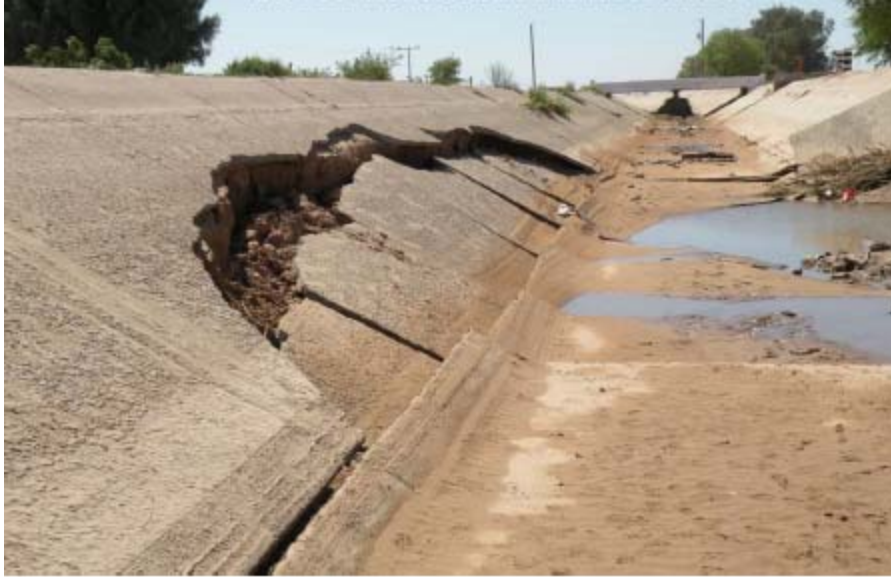
Figure 7. Slumping of embankment into the canal. Photo courtesy of CONAGUA.
