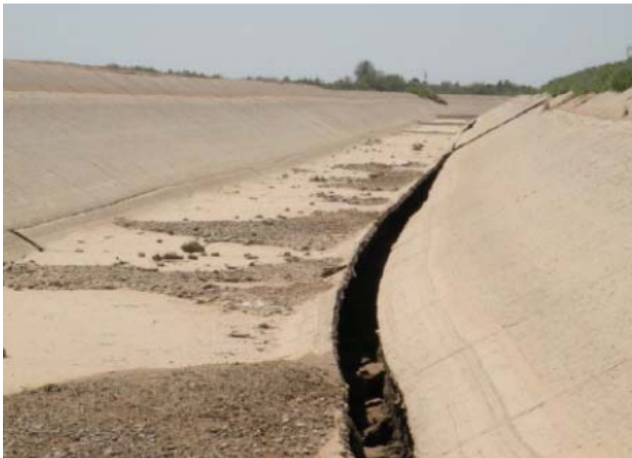
Figure 8. Movement of the entire canal embankment away from the canal. Photo courtesy of CONAGUA.
