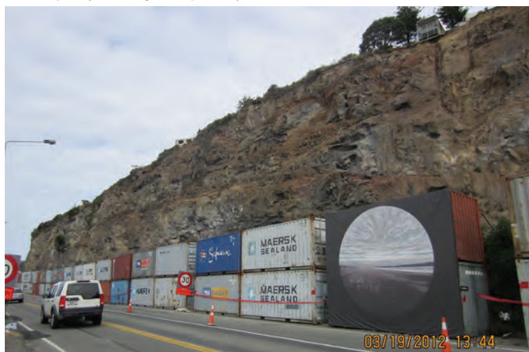
Figure 4: East Hill Area of Greater Christchurch, landslide and land deformation damage. Note the use of shipping containers as temporary retaining wall. (photo by the author)
