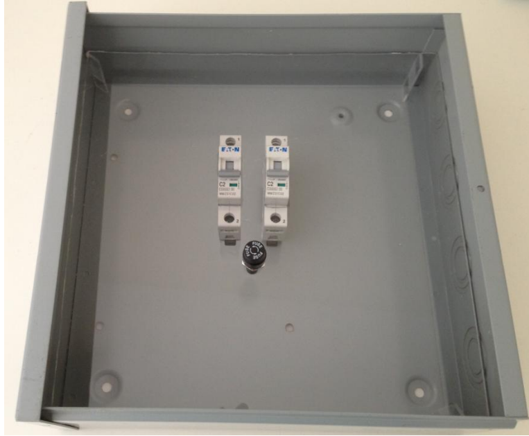
Figure 3-6: Final Layout in Distribution Panel with Components
