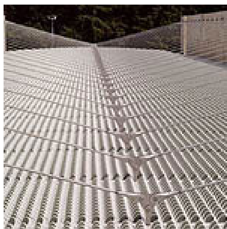
Half a million shell forms make up the Nasher roof designed by Arup. Photographer: Michel Denancé http://www.architectureweek.com/2004/0310/building_1-2.html
