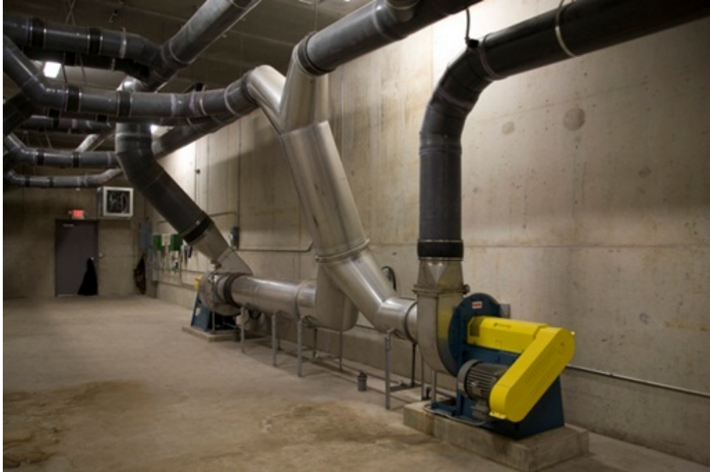
Figure 9: Fan room for SV Composters (ECS, 2015)
