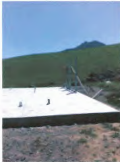
Figure 27: Pump pad at Nelson Reservoir (Kloepper, 2014)
