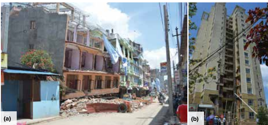
Fig. 3: Buildings damaged in the 2015 Nepal Earthquake: (a) low-rise building (after Reference 18, licensed under CC BY-SA 3.0); and (b) high-rise building (after Reference 19, licensed under CC BY-SA 3.0)
