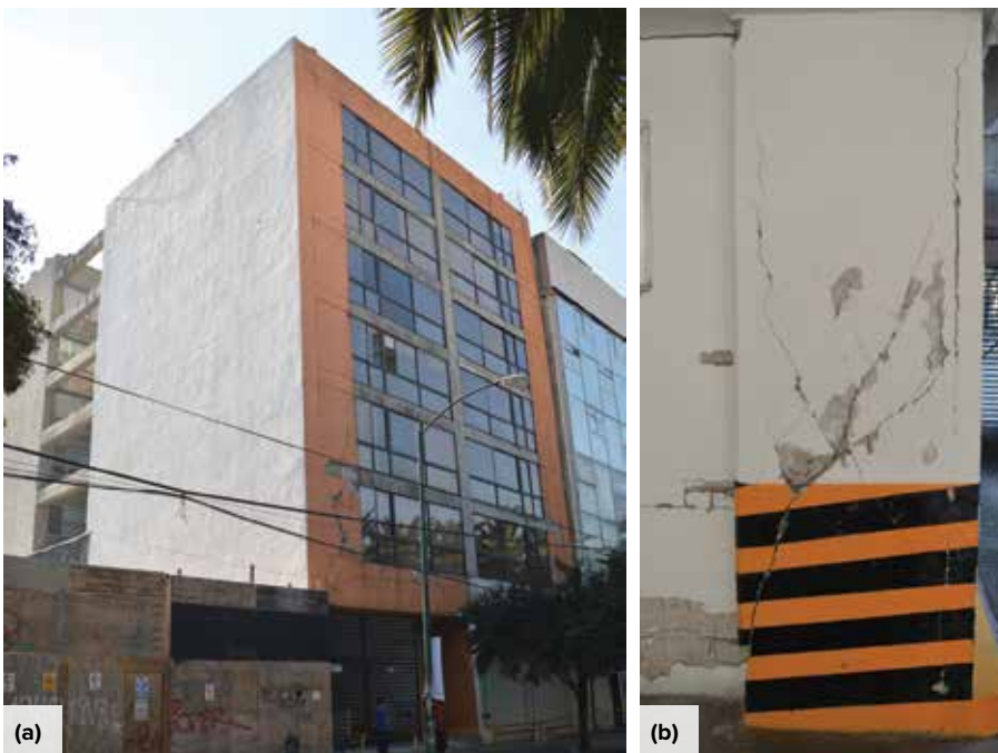
Fig. 6: A typical residential building affected by the 2017 Puebla Earthquake: (a) edge frames oriented perpendicular to the street had continuous infill walls and exhibited no significant damage; and (b) edge frames oriented parallel to the street had infill walls and fenestration and exhibited shear failure in first-story columns (after Reference 26, licensed under CC BY-NC-SA 4.0)
