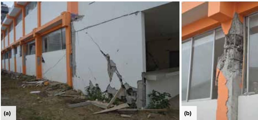
Fig. 5: Damage caused in two buildings by the 2016 Ecuador Earthquake: (a) shear failures in masonry infill walls; and (b) shear failure in a short, ground-level column above infill walls (after Reference 23, licensed under CC BY-SA 3.0)
