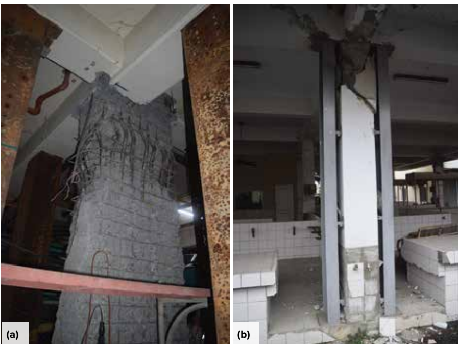
Fig. 4: Damage to columns in the 2016 Taiwan Earthquake: (a) axial compression failure; and (b) shear failure (after Reference 22, licensed under CC BY-NC-SA 4.0)
