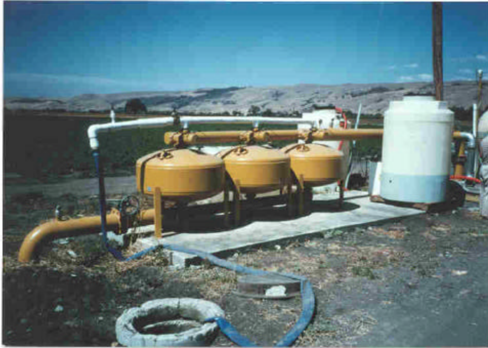
Figure 3-1. Sand media filter installation.
