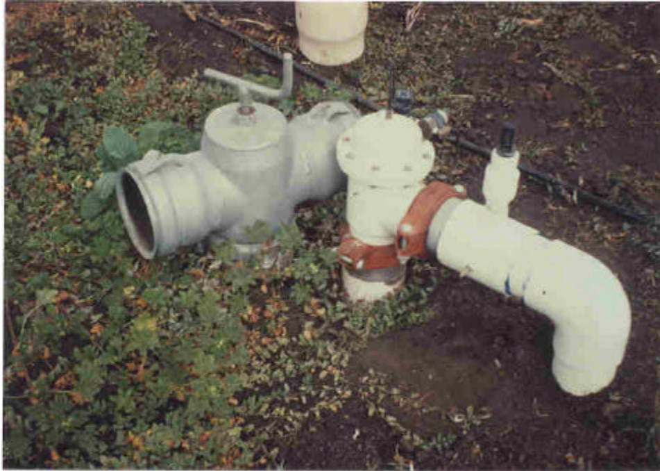
Figure 3-3. High Rise - Pressure regulator next to a sprinkler valve and riser. This model of pressure regulator was incapable of maintaining the desired pressure.
