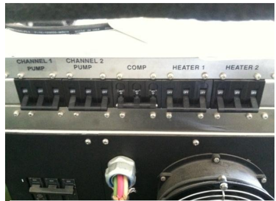
Figure 21. Circuit Breakers for Pump 1, Pump 2, Compressor (Comp), Heater 1, and Heater 2
