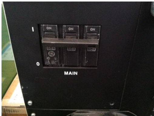
Figure 20. Main Circuit Breaker
