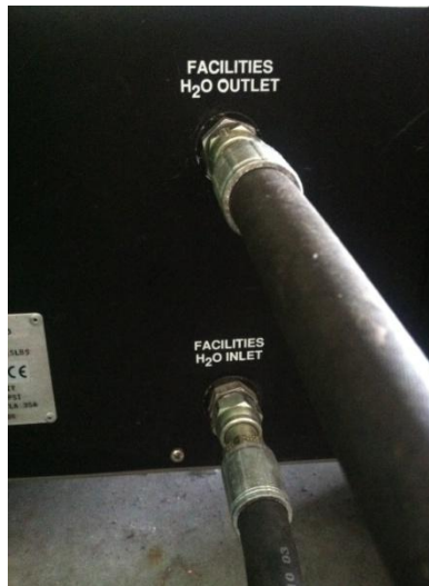
Figure 19. Facilities H2O Outlet and Facilities H2O inlet
