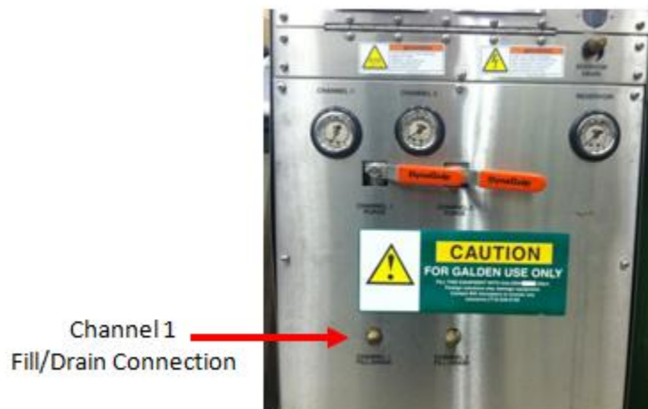
Figure 24. Fill/Drain Connection on Front of Chiller
