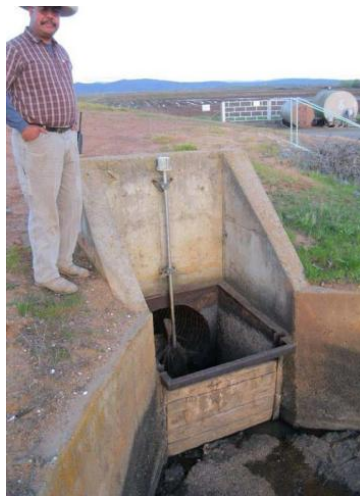
Figure 5. Propeller meter at Cordua Irrigation District (Styles, 2012).
