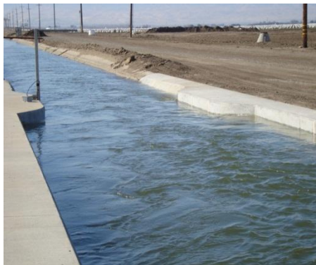
Figure 8. Subcritical Device located at the head of a main supply canal at Banta Carbona Irrigation District. Picture was taken during BRAE 533 field trip during winter 2012.
