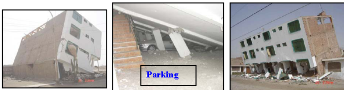
Figure 21. Collapse of a four-story confined masonry building in the 2007 Pisco, Peru earthquake (San Bartolomé and Quiun, 2008).
