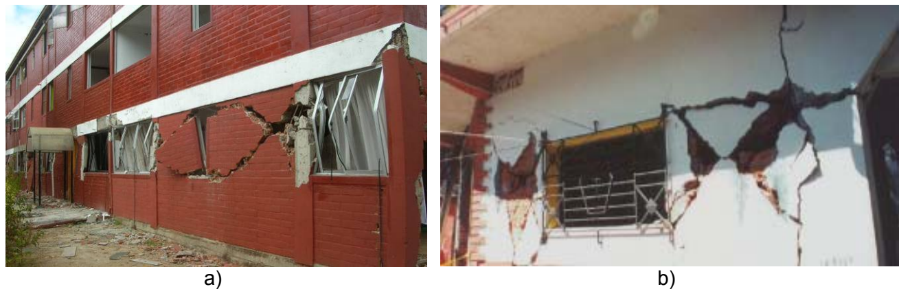
Figure 12. In-plane shear failure of poorly confined masonry walls: a) the 2010 Maule, Chile earthquake (M. Astroza), and b) the 2001 El Salvador earthquake (EERI, 2001).
