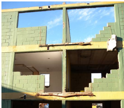
Figure 26. Absence of RC tie-columns at openings (Brzev et al., 2010).
