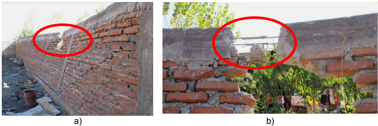
Figure 17. Collapse of a confined masonry fence in the 2010 Maule, Chile earthquake due to out-of-plane seismic effects: a) collapsed fence showing the RC tie-beam failure, and b) detail of RC tie-beam showing excessively short lap splice length in the longitudinal reinforcement (M. Astroza).
