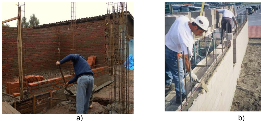
Figure 2. Masonry building technologies: a) confined masonry construction in Chile (S. Brzev), and b) reinforced masonry construction in Canada (B. McEwen).
