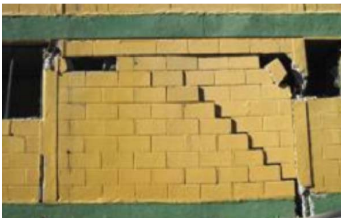
Figure 8. Critical regions in a confined masonry building: a) a general diagram showing critical regions in the RC tie-columns, and b) tie-column damage observed in the 2010 Chile earthquake (M. Astroza).
