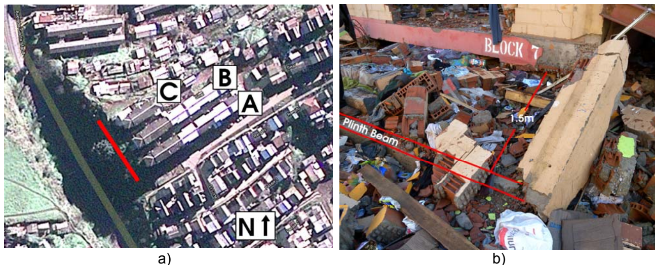
Figure 20. Collapse of a three-story confined masonry building in Constitución, Chile due to the February 2010 Maule earthquake: a) an aerial view of buildings A, B and C (note a steep slope on the north-west side shown with a solid line), and b) building C (located closest to the slope) lost the ground floor and moved by approximately 1.5 m away from the plinth towards north (S. Brzev).
