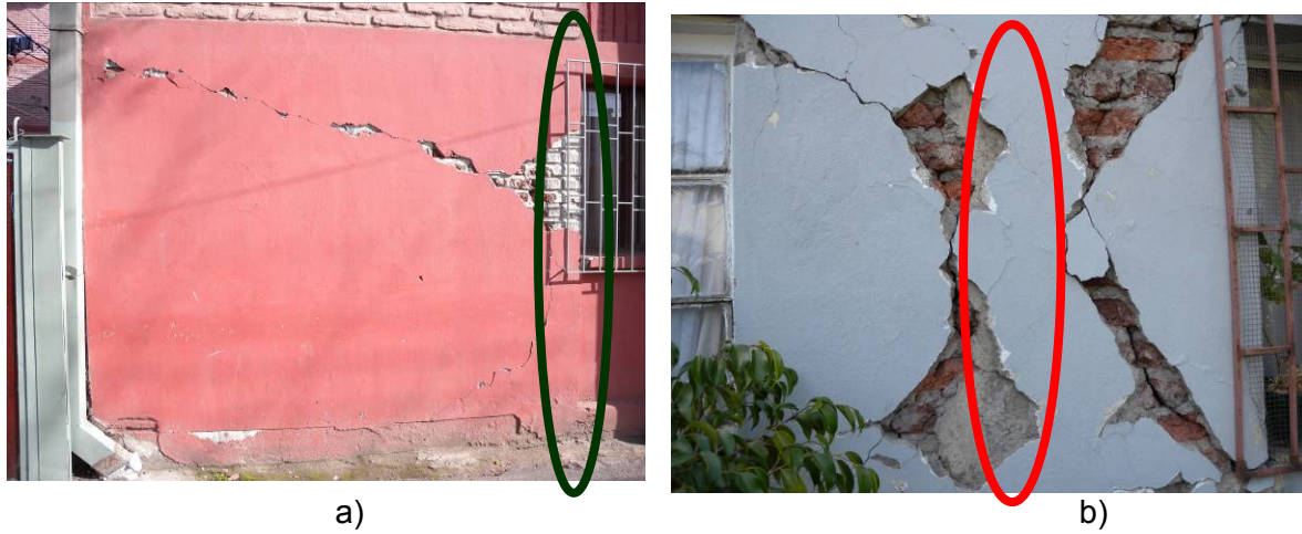
Figure 27. In-plane shear cracking of piers in confined masonry walls: a) a confined masonry panel with RC tie-columns at both ends (note RC tie-column highlighted with a black ellipse), and b) unconfined opening (note RC tie-column at the middle of the pier highlighted with a red ellipse) (Brzev et al., 2010).
