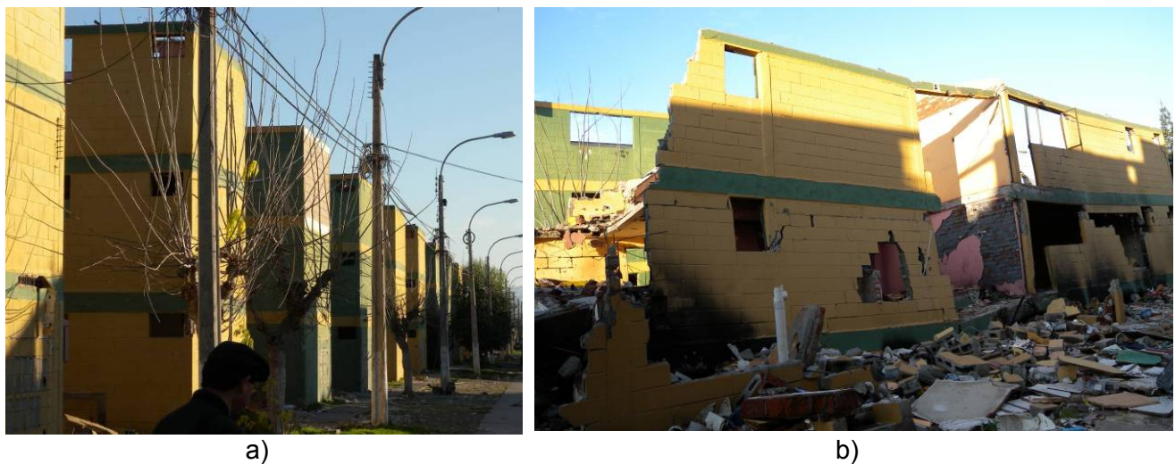
Figure 19. Collapse of a three-story confined masonry building in Santa Cruz, Chile due to the February 2010 Maule earthquake: a) building complex, and b) a building that experienced collapse at the ground floor level (S. Brzev).
