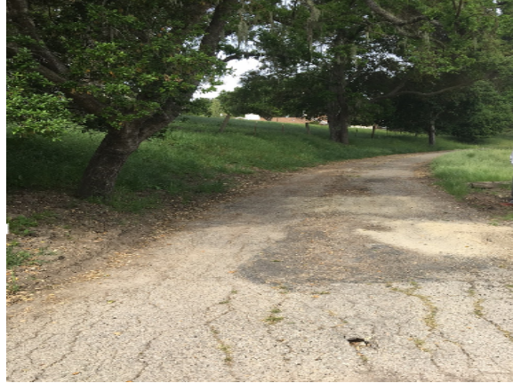
Figure 6. the damaged section of the drive for the asphalt replace project
