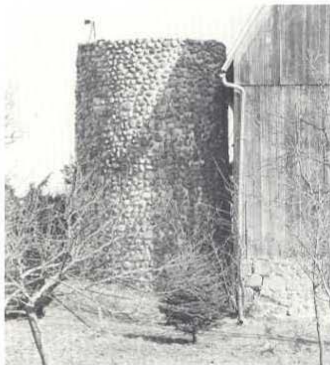
Figure 2: Rubble walled stone silo missing its roof but still standing.
