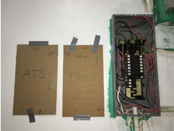
Our layout of the ATS and subpanel. This item took a few days to completely lay out to get the correct width and heights of spacing in between each item.
