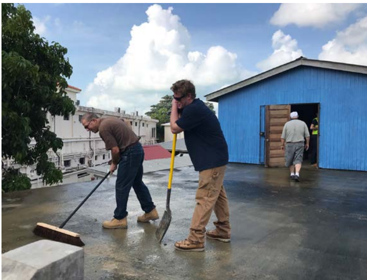
Because of the siting water, we wanted to make sure to clear out any items or liquid that was on the deck when we arrived. It took about a day to remove excess materials from the jobsite.
