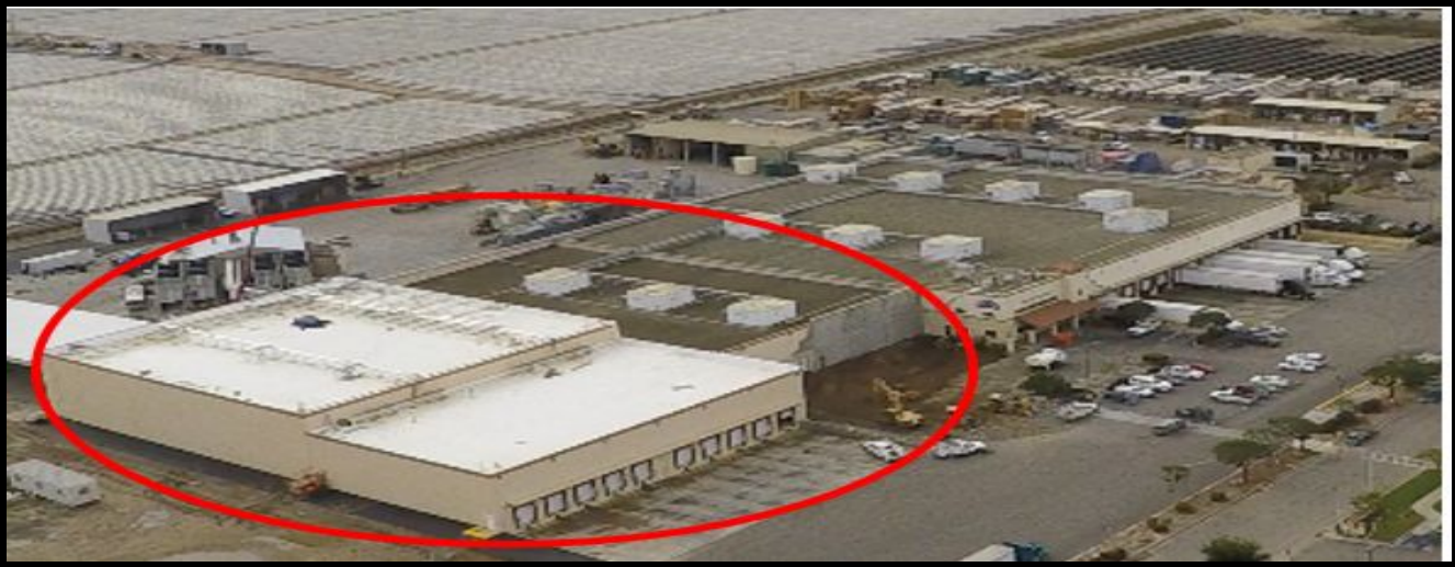
Figure 6: Bonipak Cooler Expansion
