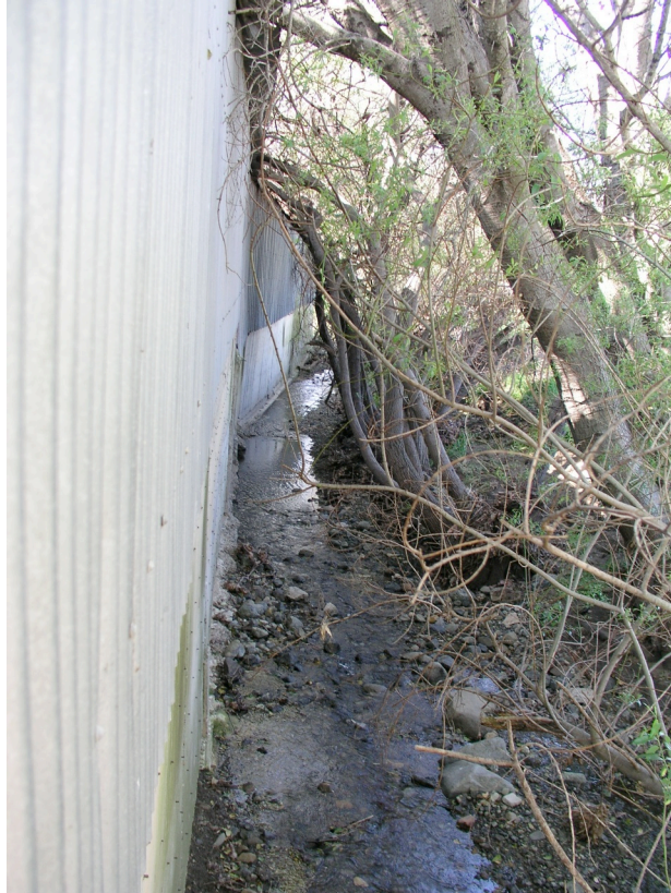
Figure 1. The Cal Poly Farm Shop forms the south bank of Brizzolara Creek prior to the implementation of the Cal Poly Farm Shop Removal and Stream Bank Repair Project.
