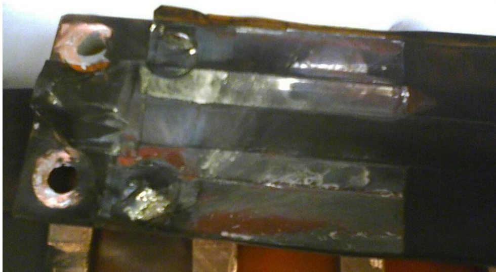
Figure 32 - Mk. 2 Internal arcing damage
