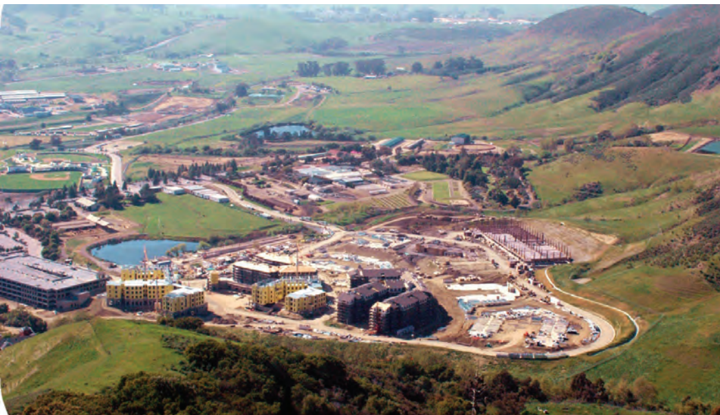
Figure 1: Poly Canyon Village. The newest student residences in the construction phase. (photo: Kevin Waldron)
