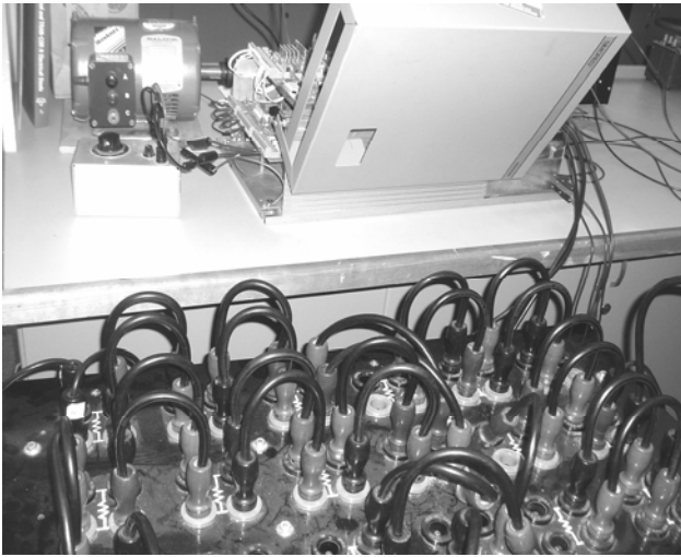
Figure 2. DC Drive (top) is connected to resistor load bank (bottom)
