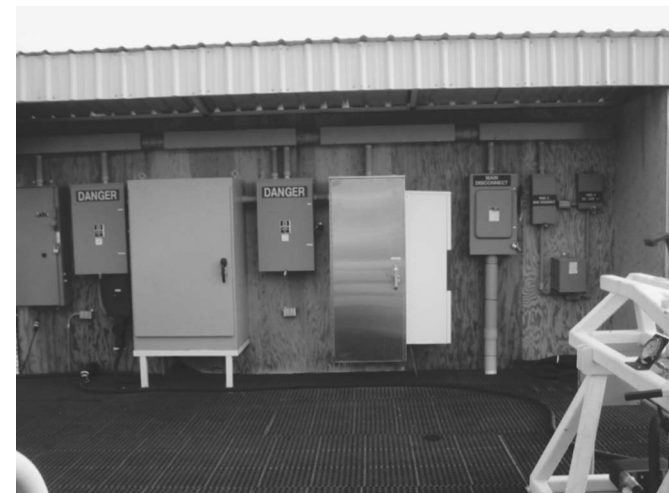
Fig. 3. Electrical supply for the motor testing
