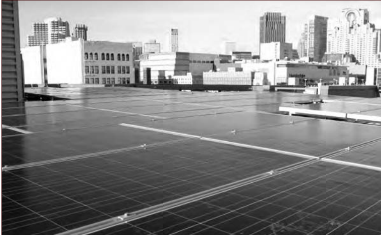
Figure 1 Solar cells at Plaza Apartments, San Francisco.
