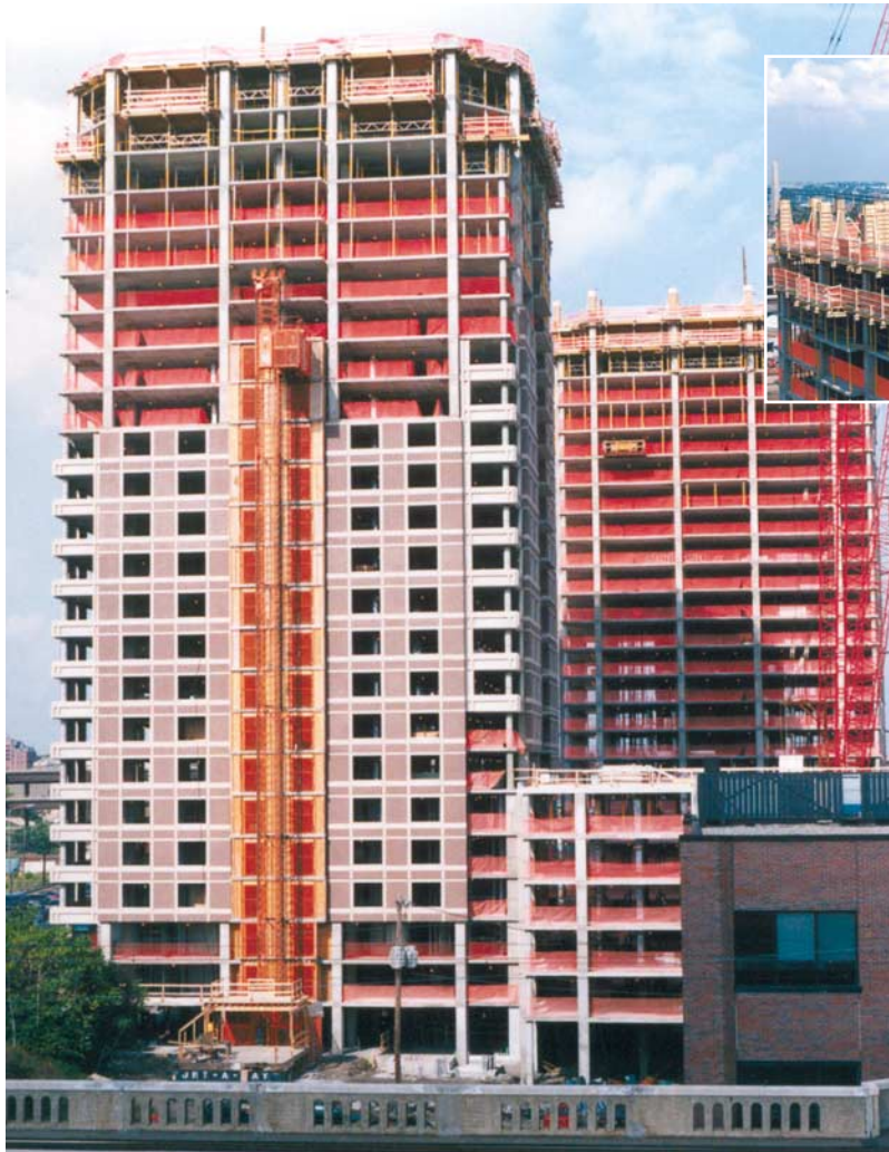
Figures 1 and 2: The construction of Museum Towers, Cambridge, Boston in 1997 demonstrated the efficiency of flat-plate slab construction.
