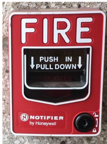
Figure 18. Notifier NBG-12LX Manual Pull Station
