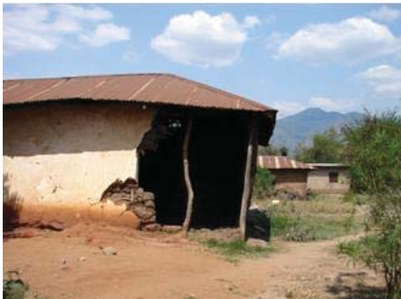
Figure 5: Adobe Brick Water Decay Source: David Lambert
