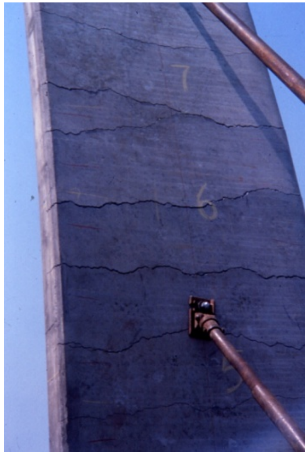
Fig. 5 – Test Panel Showing Cracking Pattern
