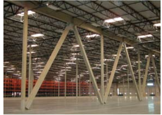
Figure 1: Large HSS shapes have been common in braced frames in the seismically active western United States. Expanding the scope of ASTM A500 will allow use of these shapes that already comply with the new seismic compactness requirements.
