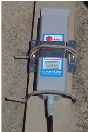
Figure 2. Unidata STARFLOW Ultrasonic Doppler Flow Meter, secured to 1/4" steel plate to anchor it on the canal floor.
