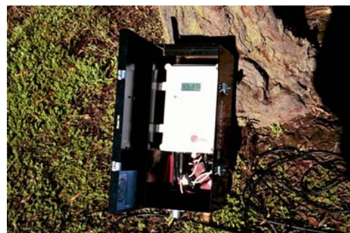
Figure 5. MicroLogger with LCD installed in toolbox for easier access, Sutter-Mutual WC.
