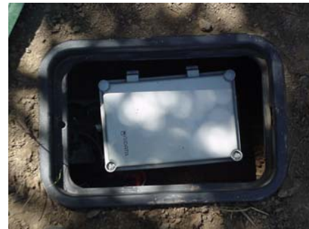
Figure 4. MicroLogger in buried irrigation valve box, Sutter-Mutual WC. The unit sits on a masonry brick to keep it off the ground.
