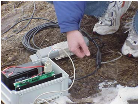
Figure 3. STARFLOW sensor connected to MicroLogger box, Kittitas ID. Note the battery and the communications cable connecting the MicroLogger to a laptop computer.
