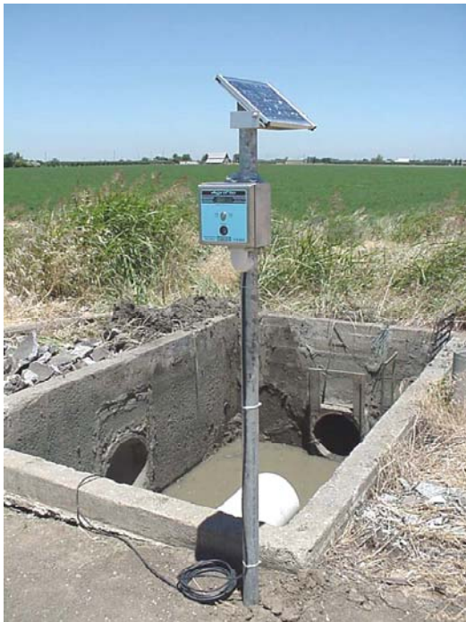
Figure 6. The MACE Agriflo Doppler Flow meter installed at Patterson Irrigation District
