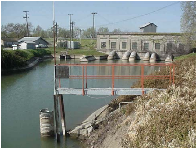
Figure 2. Tisdale Pumping Plant
