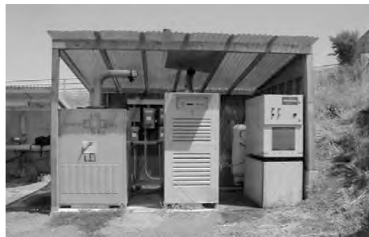
Figure 5 – Cal Poly 30kW Microturbine Installation After Williams, D.W. and D. Gould-Wells, 2003
